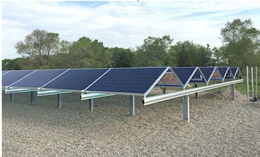
Runestone Electric Association 44 KW Community Solar Alexandria, Minnesota
