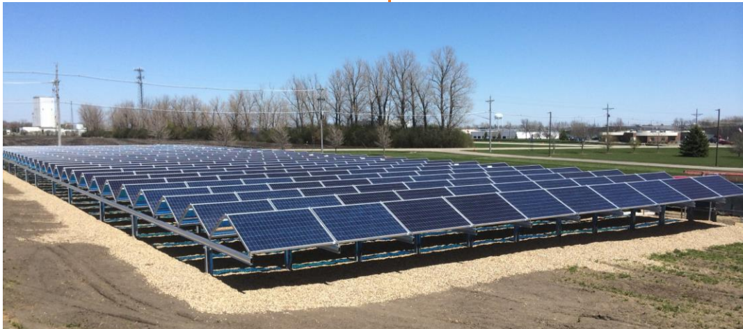
Steele-Waseca Cooperative Electric 100 kW Sunna Community Solar Garden Owatonna, Minnesota
