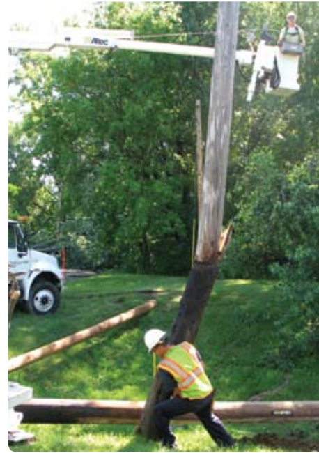
Dozens of broken poles needed to be replaced.
